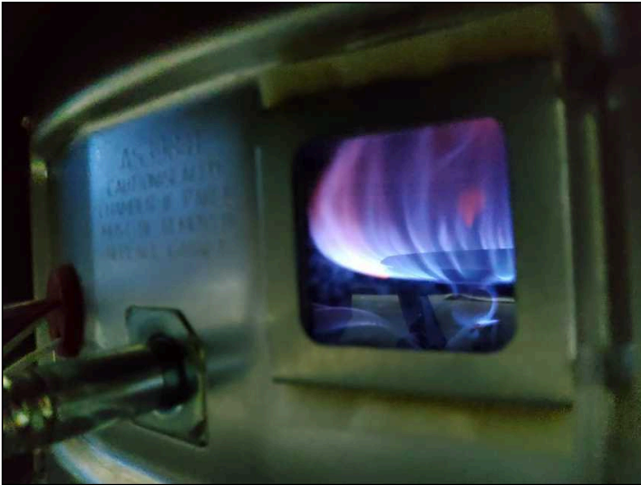
Combustion chamber can only be partially inspected, rust and scale noted - On going monitoring required.
