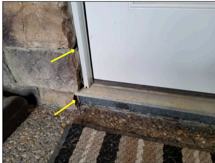
Missing and split caulking observed, recommend resealing as part of the ongoing maintenance
