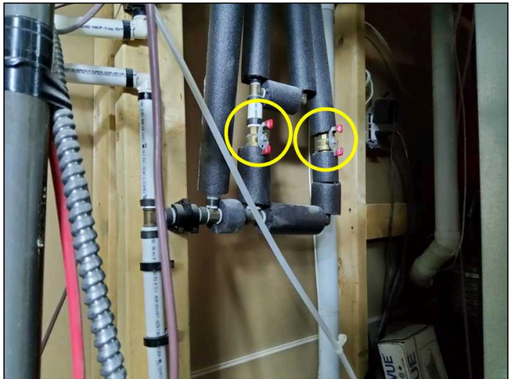
External faucet shut off valve circled
