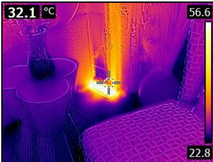
Living room heating register, responding to test
