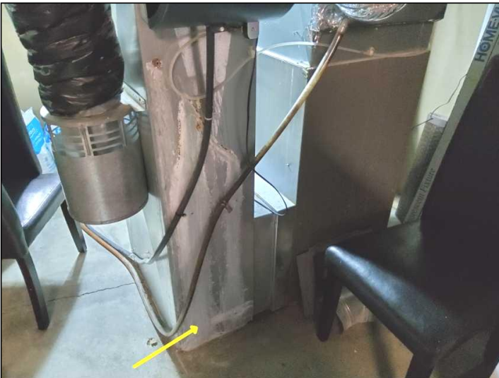
Rust and corrosion noted to the housing of this unit. Recommend inspection by a qualified HVAC contractor.
