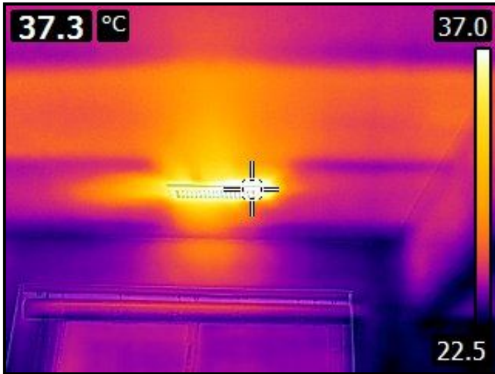
Basement bedroom heating register, responding to test
