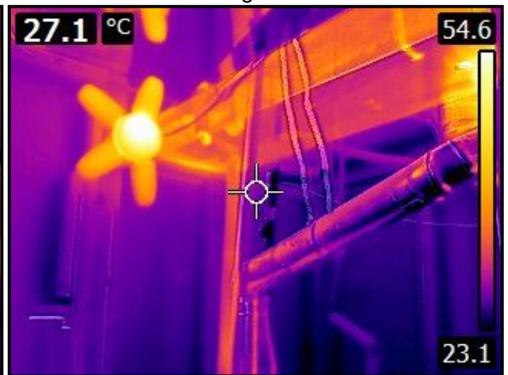
Mechanical room thermal image
