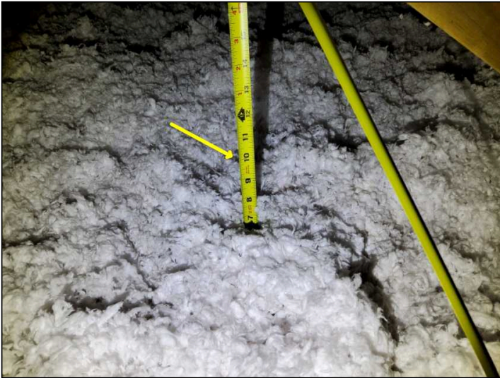
Approx 8-10 Inches of insulation noted in the attic space - Low compared to todays standards, suggest adding more to reduce heat loss.
