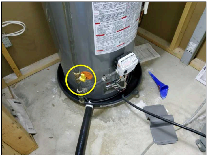
Gas shut off valve circled
