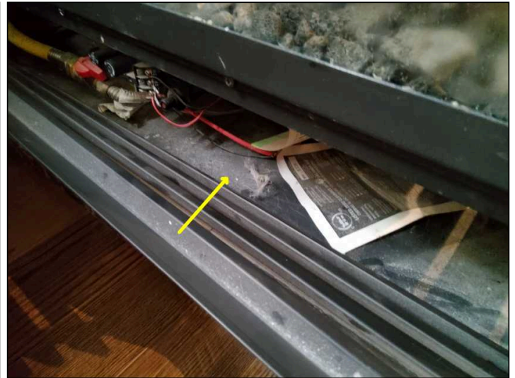
Recommend servicing and cleaning by a contractor.
