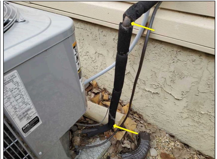
Deterioration noted to the insulation at the condensate line. Recommend replacement.
