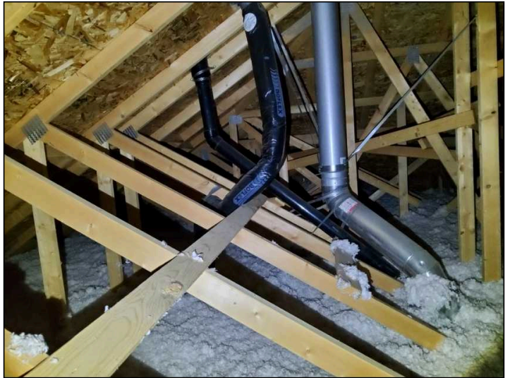
Unable to determine condition in some areas due to framing and insulation cover.
