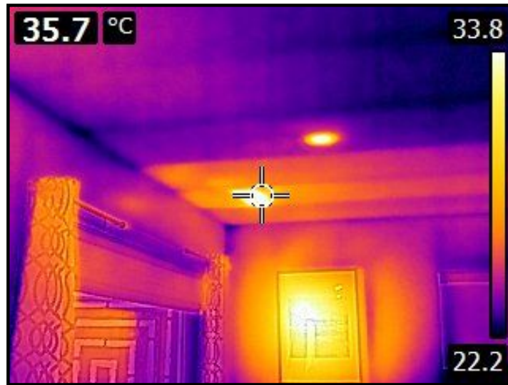
Basement heating register, responding to test
