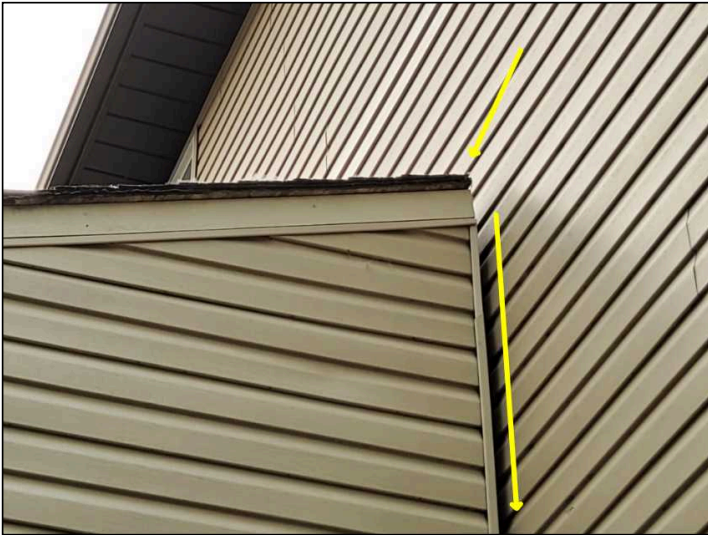
Recommend installing a flashing at side shed to siding, to help prevent moisture seepage down to foundation and moisture intrusion into shed. Limited inspection recommend further review
