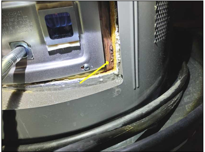
Rust and scale noted to combustion chamber
