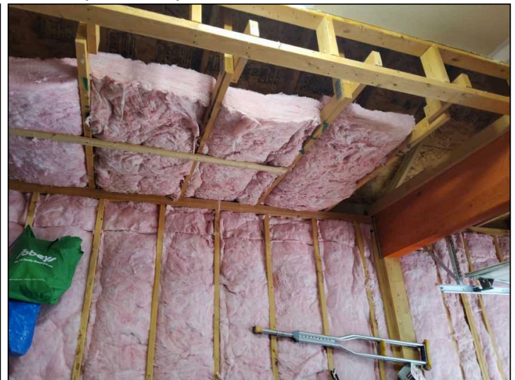
Garage partially insulated, loose insulation noted, Missing vapour barrier observed, recommend review for repair or replacement
