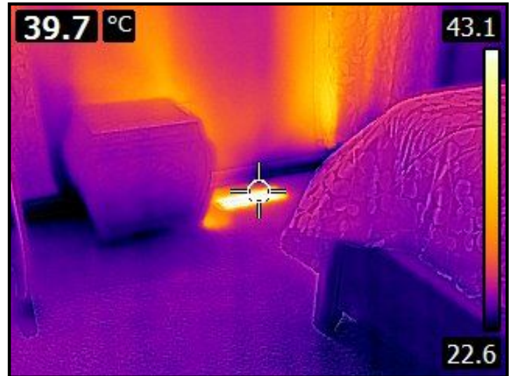
Bedroom heating register, responding to test.
