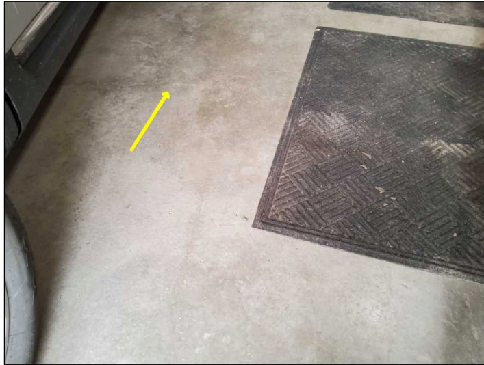
Cracks and settling observed, suggest sealing cracks as necessary.
