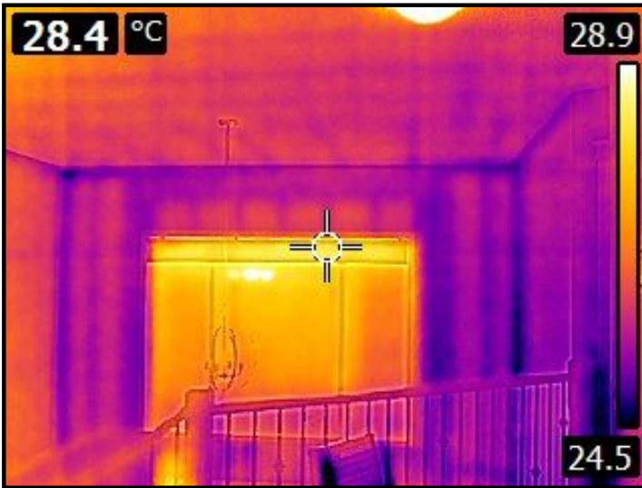
Upper landing thermal image
