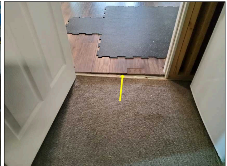
A sub floor has been added. Unable to inspect the original slab.
