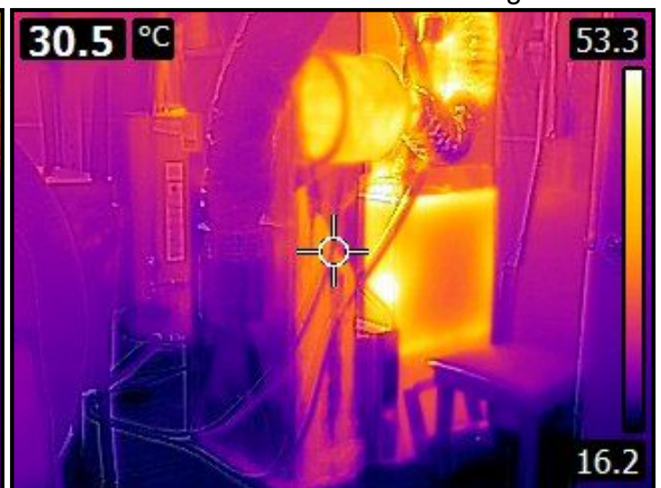
Mechanical room thermal image
