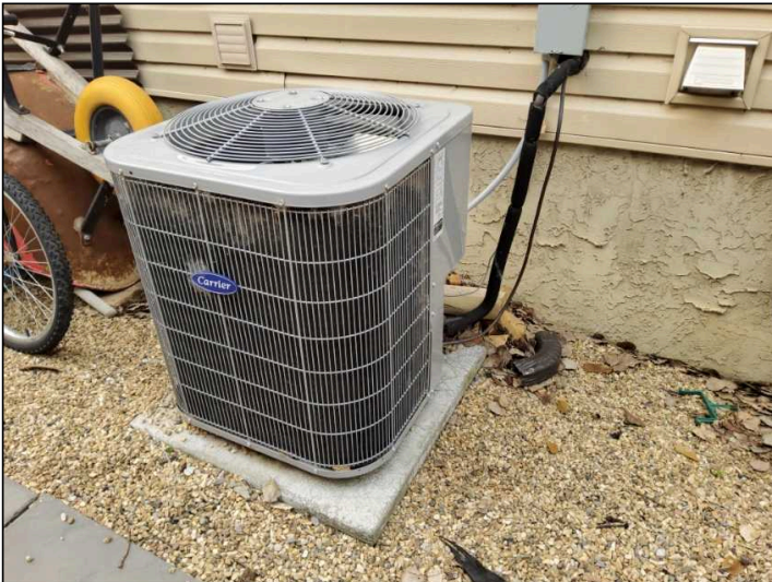
Tested and working on day of inspection - Please only activate or test when external temperature is above 16 degrees, operating at lower temperature can cause internal damage to unit.
