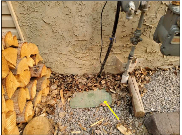
An automatic sprinkler/irrigation system was observed but not inspected or tested. This system is beyond the scope of this inspection. We recommend further review by a qualified professional, if desired.
