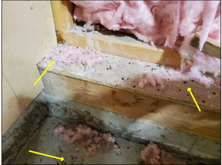
Indication of possible pest activity observed, recommend further review by a certified pest control if concerned
