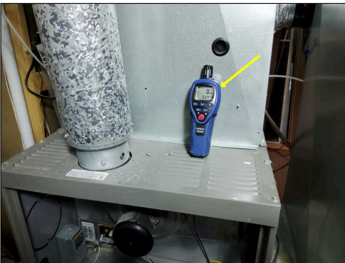
Carbon monoxide reading was ZERO during inspection.
